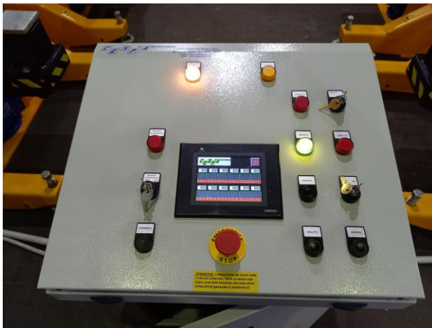
MAIN INDEPENDENT CONTROL PANEL
